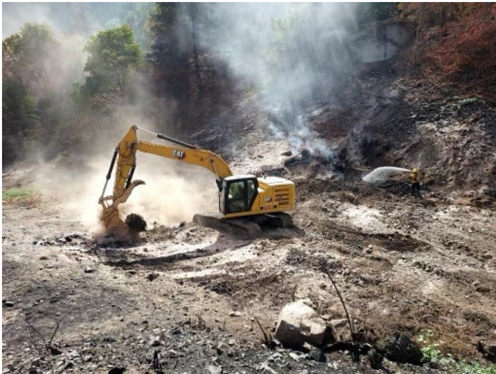
Photo: An excavator works in the waste disposal pit alongside a firefighter. USDA Forest Service photo by Josh Voshall, Mt. Hood National Forest.
